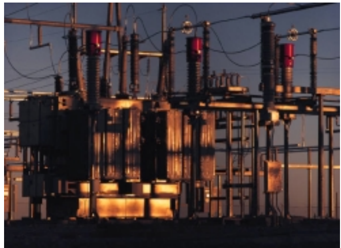
A substation may benefit from DG applications
