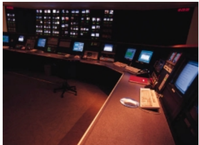
Backup systems are used to power critical loads such as this control center.
